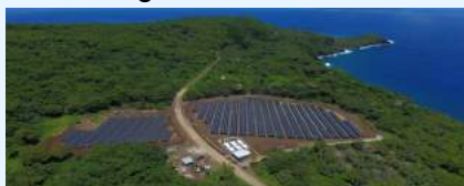
Solar panels in Manu'a, American Samoa
